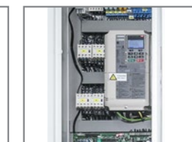
Controller MRL lift plant
